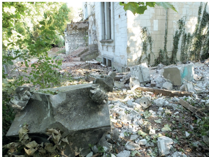
Fig. 8 Rubble around Spitzer Villa after the demolition of the roof (Photo: Predrag Komljenović 01.10. 2016)
