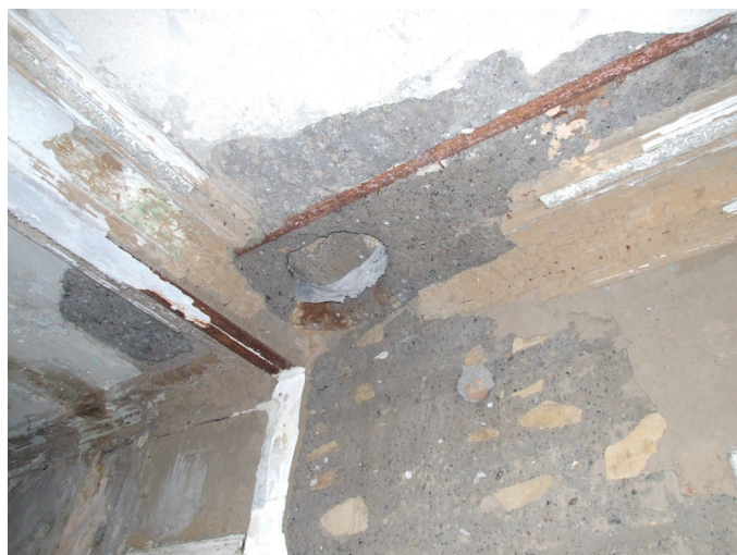
Fig. 6 Spitzer Villa – concrete wall and ceiling on the second floor (Photo: Viktorija Aladžić 2014)
