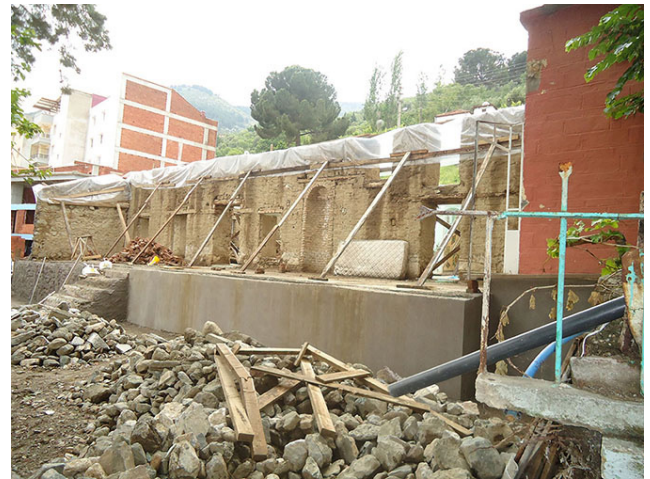
Fig. 3 Adobe mud-brick masonry walls with timber lintels, Haki Baba Mosque, during the 2014 restoration application
