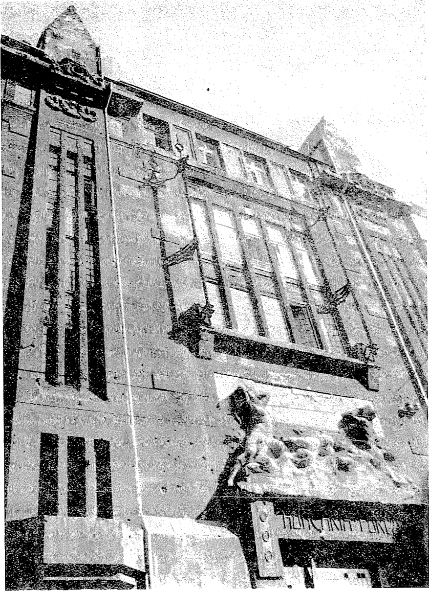
Fig. 14. Swimming pool of Hungaria Bath. Detail of the façade. Actual condition
