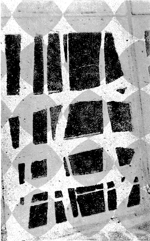
Fig. 8. Detail seen from outside of the glass-concrete window of the Bagatelle church
