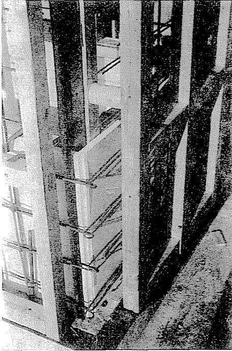
Photo 14. Erection of U-section pillars: mounting the auxiliary frames. Close view. Lower corner detail: inner element and reinforcement positioned. Erection of pillar starts with the assembly of auxiliary timber frames whereby the position of each surface of the pillar is exactly determined. Accuracy required from thin r.c. folded shell structures was provided by using simple cylindrical spacers. The pillar is built of six rows of units of a height 6 M = 60 cm. This basic repetitive cycle is composed of two main phases: 1. the assembly of surface (negative mould of the load-bearing structure) a) placing inner surface elements; b) positioning of reinforcement; c) placing outer surface elements; 2. pouring in concrete resulting in the actual r.c. folded shell structure
