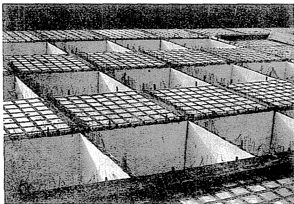
Photo 26. The tissue-structural top-of-cell units are placed by rows in the sequence shown. The units rest first on the protruding reinforcing wires. The channels formed between adjacent floor units are filled out with concrete, whereby the tissue becomes a one-way continuous structure
