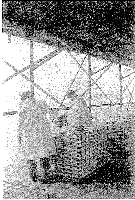
Photo 11. Concreting polystyrene-gypsum floor units. The dry and hardened floor units are sorted according to types and concreted superimposed in stacks. The units are separated from each other by corrugated cardboard sheets. The r.c. tissue arises from pouring concrete into the two-way channel system
