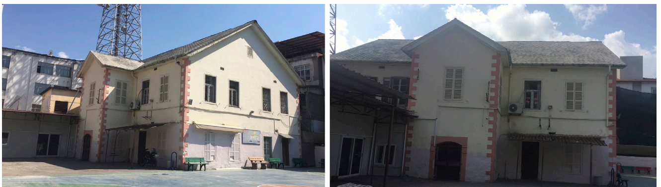
Fig. 5 North and west facades of the historical building visible from inside the school courtyard (Source: Authors' Archive)
