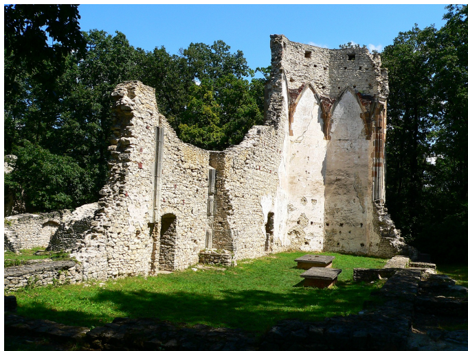
Fig. 1. The current condition of the church
