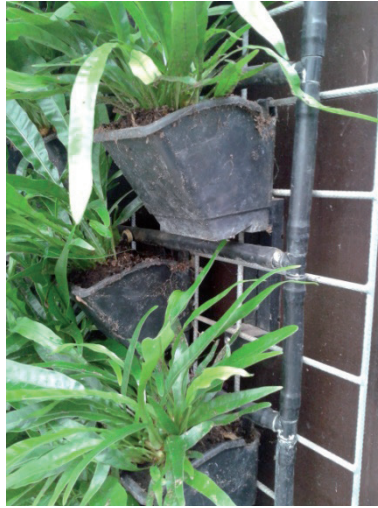
Fig. 8 Irrigation pipeline is provided on every level
