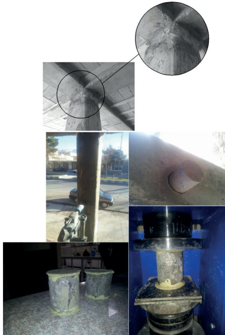
Fig. 3 View of the poorly constructed connection and the core extraction operation
