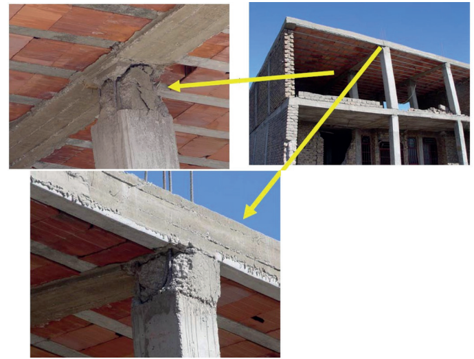
Fig. 2 Damage and rotation inflicted upon the end of the columns of a building by the 2003 Bam earthquake, Iran
