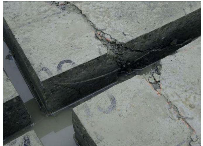
Fig. 25 Concrete center slab G04 - Crack (detail)
