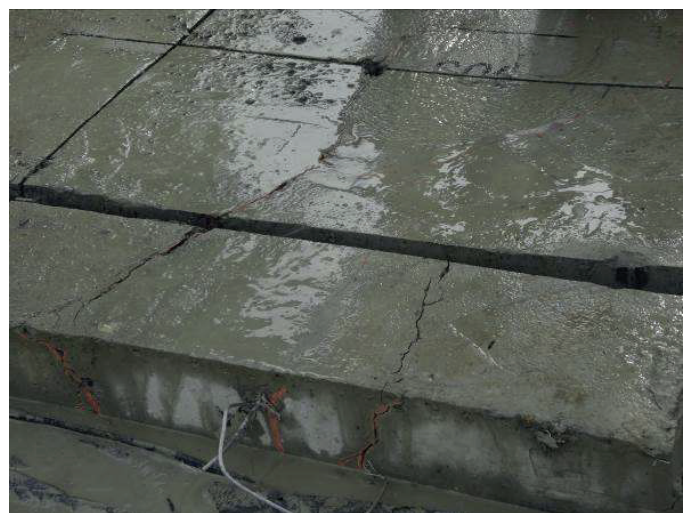
Fig. 22 Concrete edge slab G04 - Crack (Detail)
