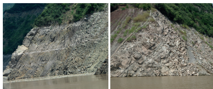
Fig. 1 Typical failure of the sandstone rock mass in the vicinity of hydro-fluctuation belt (Three Gorges reservoir area, 2015)
