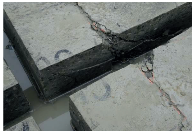
Fig. 4 Concrete center slab G04 – Crack [3]
