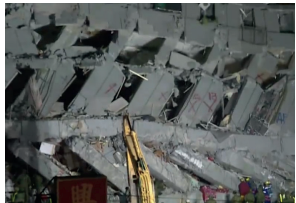
Fig. 1 On the pictures, we can see the frameworks of the demolished buildings without diagonal braces. In the top picture, a wooden framework, that lost their walls as braced elements at the 1995 Kobe earthquake (photo by Michio Miyano) [62]. In the picture below we can see the side view of the building that lays on its front side at 2016 earthquake Tainan, southern Taiwan (captured picture from [63]). We can see both of the cases the shear deformation of the structure
