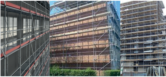
Fig. 3 We can see the three scaffolding frameworks with the largest displacements that possible in the lateral direction if we use the same number or diagonal braces
