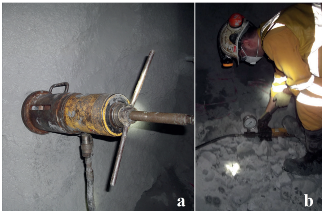
Fig. 7 Pull out test: a) bolt pulling, b) loading by using the jack handle
