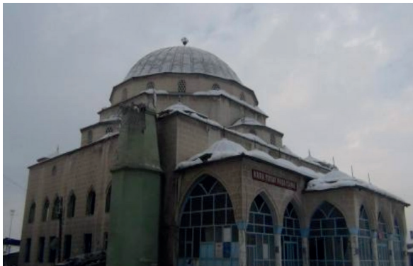
Fig. 6 Heavy damage on minaret located in Van [12]
