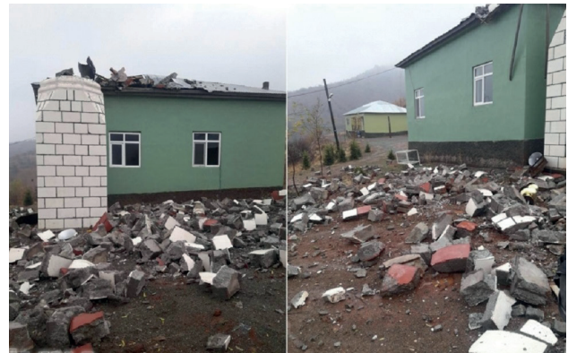
Fig. 4 Demolished minaret located in Ulubey [10]
