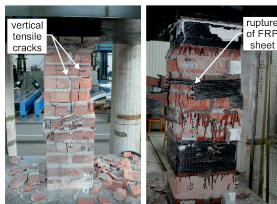
Fig. 4 URM and RM column's failure
