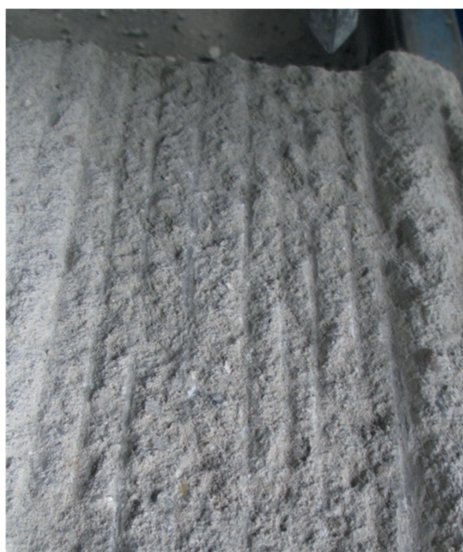
Fig. 4 Original damaged rock surface before cutting
