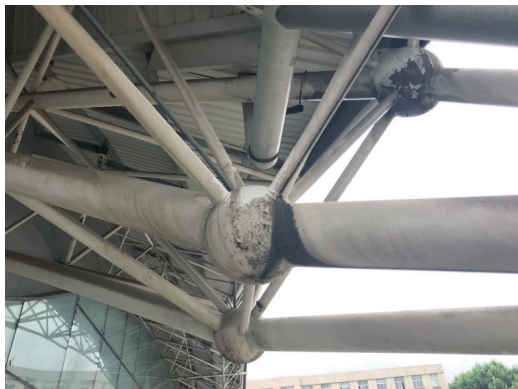
Fig. 2 Corrosion in the joints in steel structures
