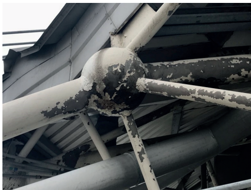
Fig. 1 Corrosion of a welded hollow spherical joint
