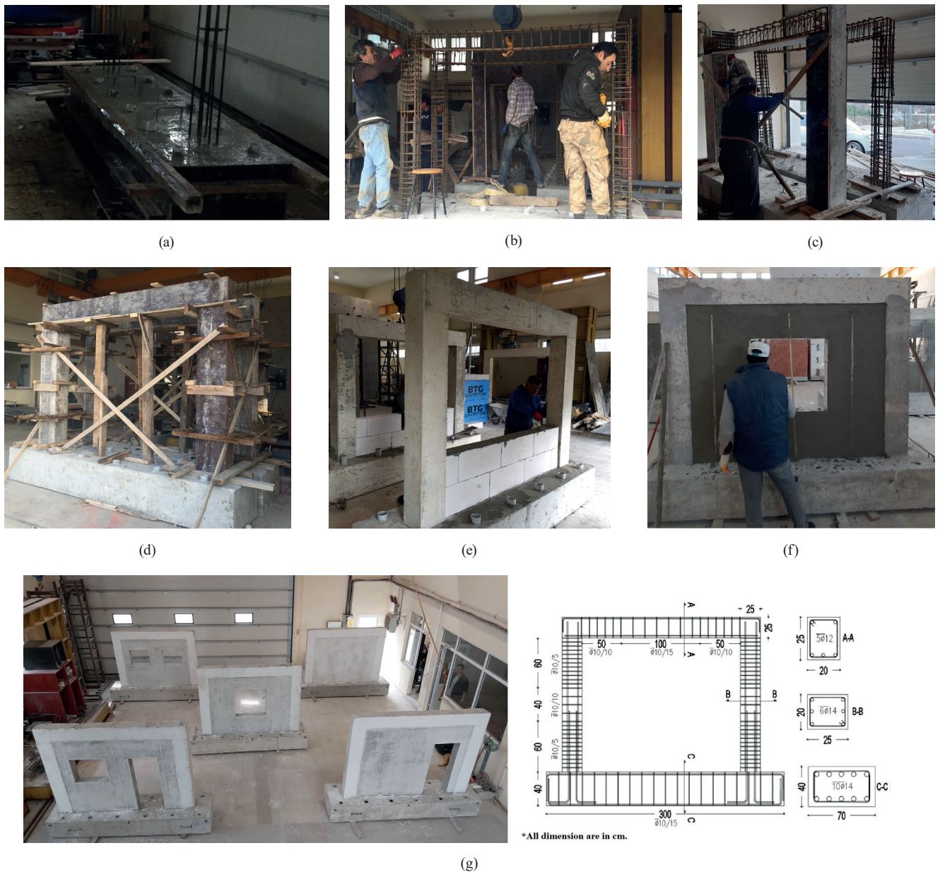
Fig. 1 Production stages of RC frames with infill walls; (a) Preparation of foundation, (b) Preparation of rebars, (c) Preparation of mold, (d) Pouring of concrete, (e) Producing of infill wall, (f) Plastering the wall surface, (g) Dimensions and reinforcement details of the test frames
