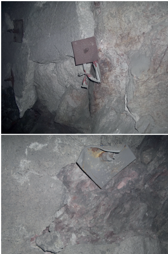
Fig. 9 Cracked shotcrete liners and bended bolt plates due to the squeezing problem of the tunnel construction
