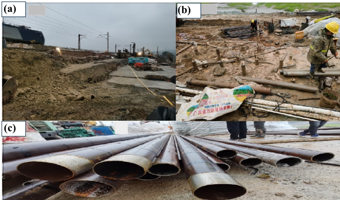
Fig. 5 (a) Failure surface (b) Grouting process (c) Steel pipe (SP) materials
