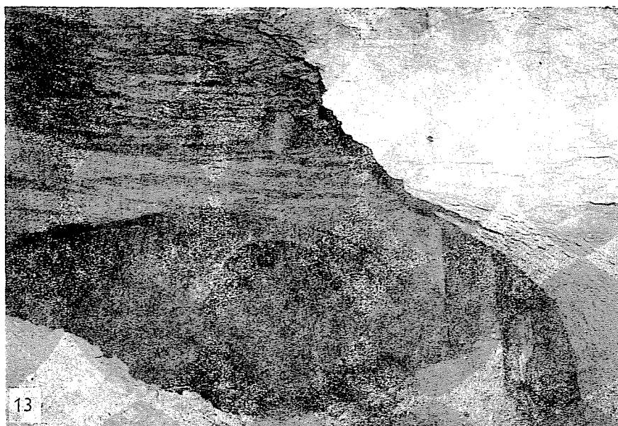
Fig. 13. Sink of a wide-span cellar roof in stratified tuff (Eger)
