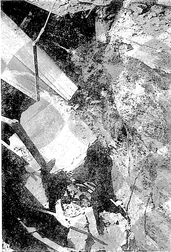
Fig. 20. Vertical rupture with building deterioration
