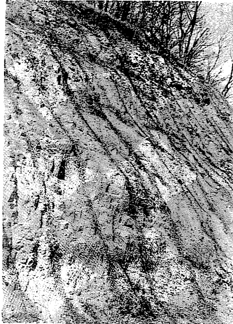
Fig. 13. An andezit surface broken with a deep slope of a road cut and protected with "nettlon" net
