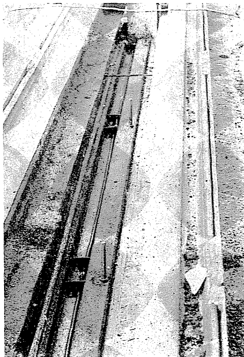
Fig. 36. Producing compressive force in the rail by heating in the direction of its longitudinal centre line
