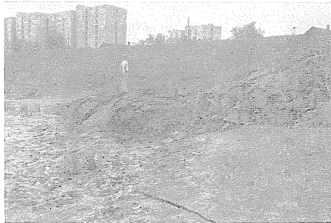
Fig. 2. The July 23, 1975 base failure: a — spot of the base failure; b — surface upheaval before the embankment foot
