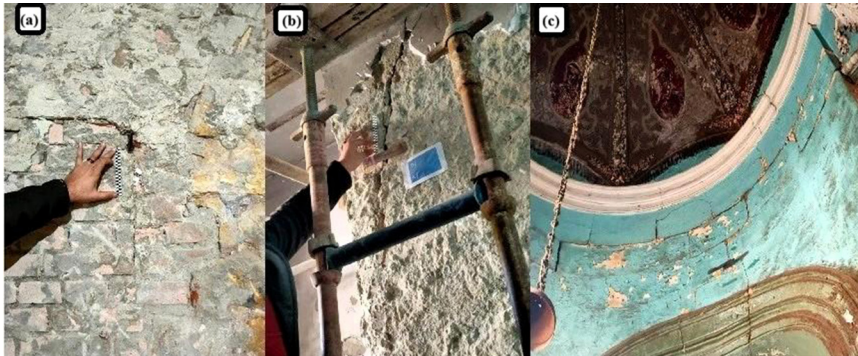
Fig. 1 Cracks observed in the case study: (a) cracks in the basement wall; (b) cracks in the first floor; (c) cracks between the blocks
