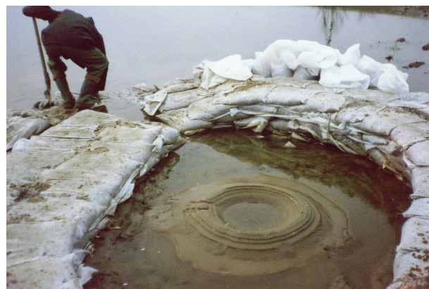
Fig. 9. Piping at Dombrád (1998), some 20 m away from the dyke toe (Area No. 3 in Tables 1 and 2.)
