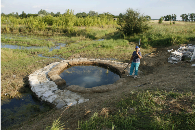
Fig. 12. Piping at the initial section of a trench drain near Tiszakürt in 2010 (Areas No. 19 – 20 in Tables 1 and 2.)
