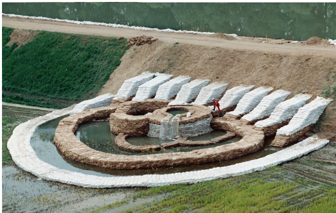
Fig. 1. The giant piping at Tiszaszas in year 2000
