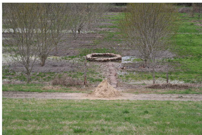
Fig. 5. Piping at Dombori as seen from the crest of the dyke. Washing out of soil first occurred some 20 metres away from the toe of the embankment (Areas No. 5-8 in Tables 1 and 2.)
