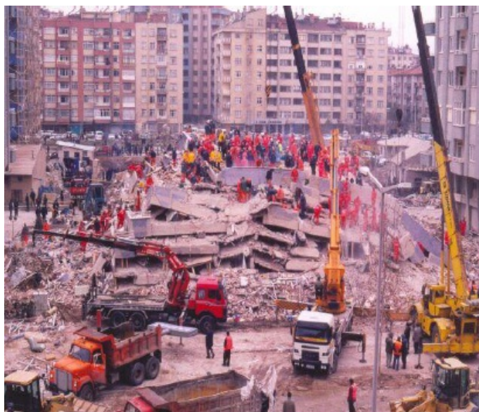
Fig. 2. Zumrut Apartment House collapsed in 2005 [9]
