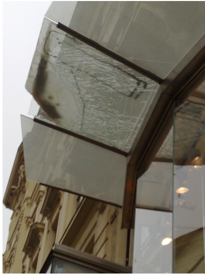
Fig. 1. Fractured overhead glazing, Humanic store, Vienna, 2007.
