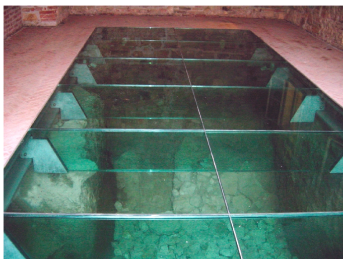
Fig. 17. Load bearing glass slab in Sándor Palace, calculations of glass and steel construction by K. Pankhardt, in 2001
