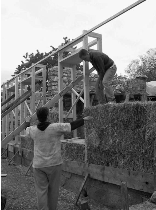
Fig. 1. Experimental work: third year students constructing the first straw-bale building in Hungary, Sáropatak
