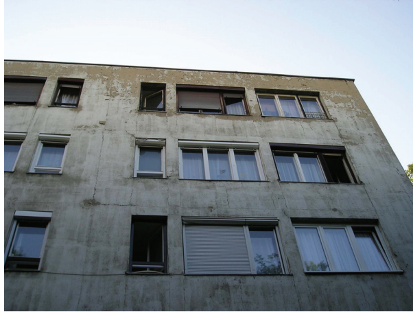
Fig. 2. Typical gaps along the blocks of a building constructed by the large block construction system.
