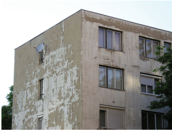
Fig. 1. Damaged facade of a building built by the large block construction system.
