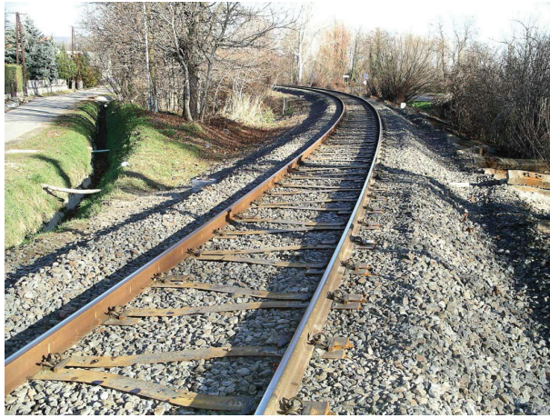
Fig. 4. The track with Y-shape steel sleepers and its surroundings at chainage of 1041 + 40
