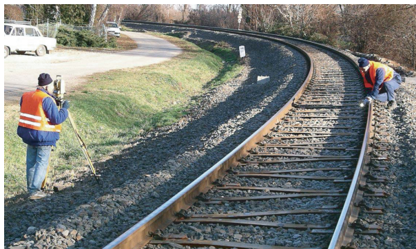
Fig. 8. Carrying out the measurement of the position of the points on the sleepers
