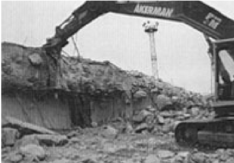
Picture 1. Remains of demolished buildings are very great in our days
