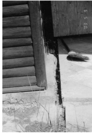
Fig. 4. Pavement next to the building came out of place
