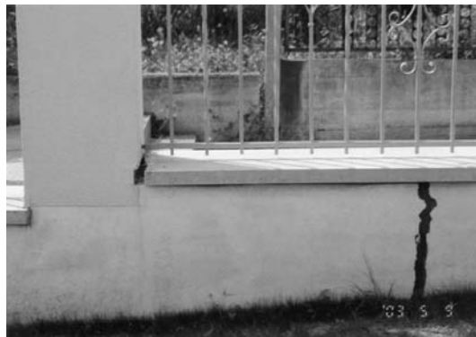
Fig. 2. Strongly marked fracture in the fence footing
