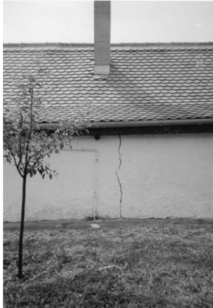
Fig. 1. Fracture on the wall of a house
