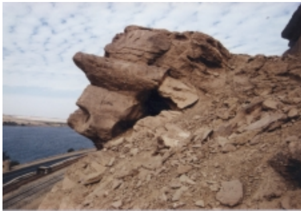
Fig. 16. A huge sliding sandstone block above the railway track, section 853+950
