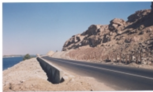
Fig. 14. Rail ‘curtain’ and reinforced concrete retaining wall at the landslide area for stabilising the highway, 853+900 section of the railway track
