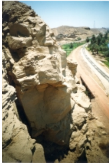
Fig. 13. Tectonised unstable cliff face at the ‘Nubian village’, section 794+220
