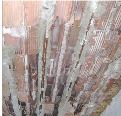
Fig. 6. Failure of bottom plane of RC slab above the false ceiling
