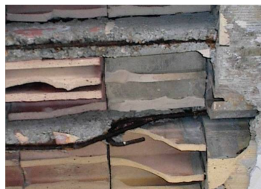
Fig. 5. Close view of the ceiling failure
