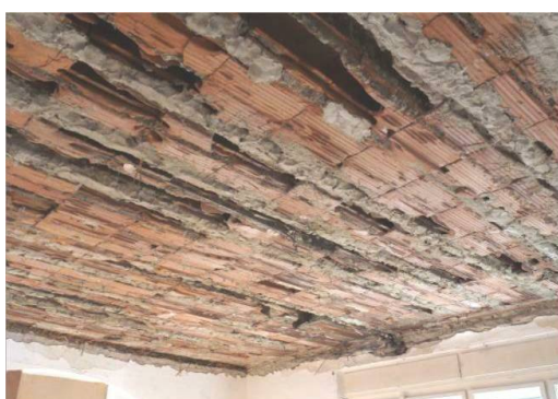
Fig. 8. Underneath view of a bigger portion of the subjected "Ujlaki" hollow block floor
