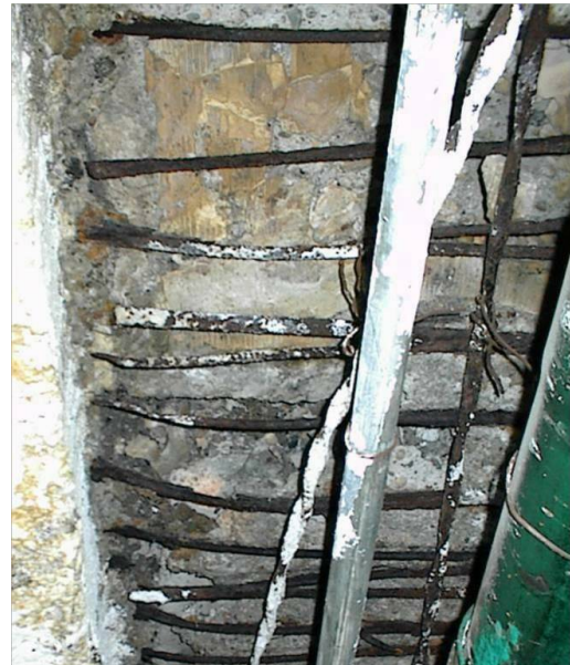
Fig. 4. Unexplainable located fired ceramic pieces above reinforcement preventing concrete to envelop rebars in an RC slab
