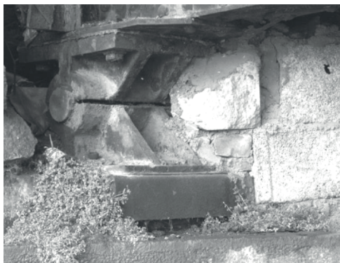
Fig. 7 Non-functional bridge bearing
