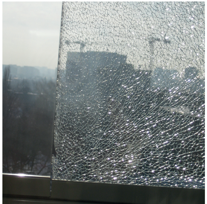
Fig. 5 Representation of the actual way of the propagation of the general stress in the glass panel, consistent with lines of cracks from the place of the initiation of the process of destruction (marked point) generated by excessive pressure of the glass panel to the metal without elastic spacers
