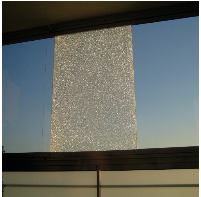
Fig. 4 One of the damaged glass panel (ESG type) mounted without elastic inserts spacing glass and metal faces of transoms of the facade system. The neighbouring panels, properly assembled, exposed to the same load, work properly
