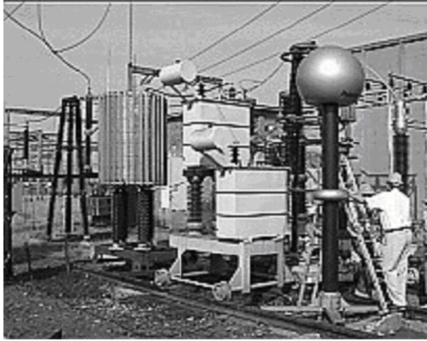
Fig. 8. One part of the HV test circuit
