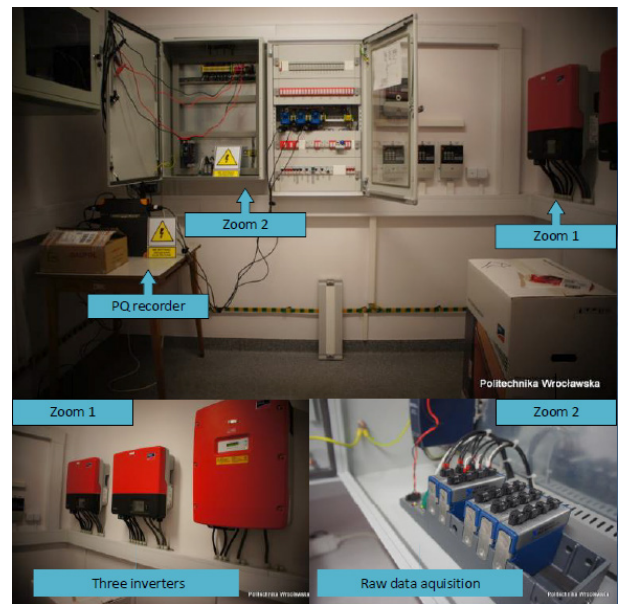
Fig. 2 The view of PV installation monitoring system at the University building [13].
