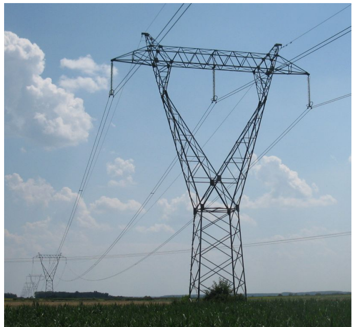
Fig. 1. High voltage overhead line
