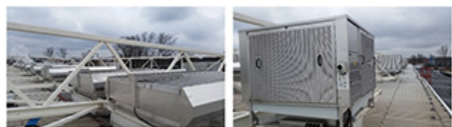
Fig. 3 Labyrinth ventilators and adiabatic coolers installed on the roof
