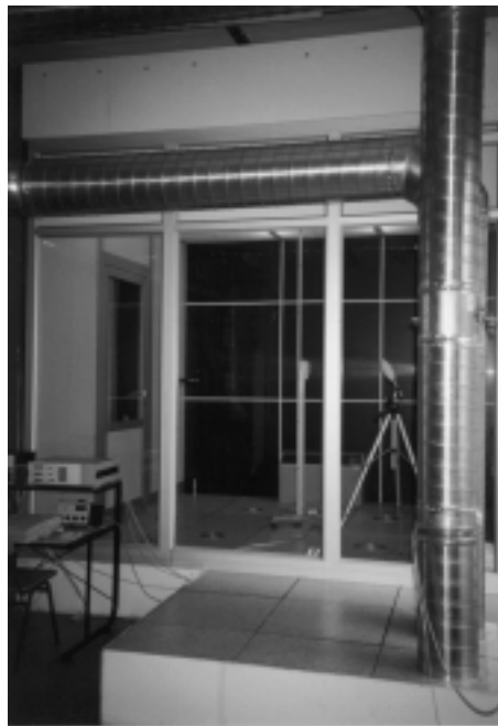
Fig. 1. Investigation chamber of air supply system
