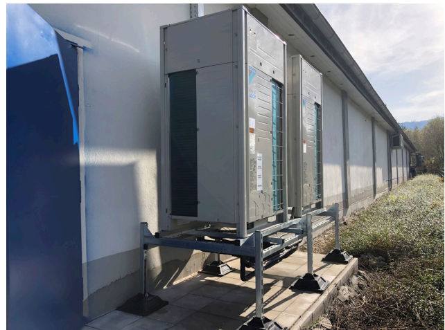
Fig. 10 Outdoor condensing units (authors' archive)
