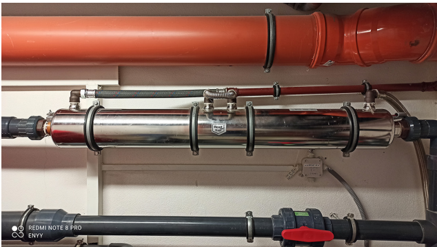
Fig. 1 Tubular heat exchanger in the engine room of the swimming pool [Authors]
