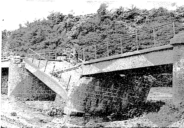
Fig. 15. Floods destroyed many a bridges on the road to Ikizdere in May 1959
