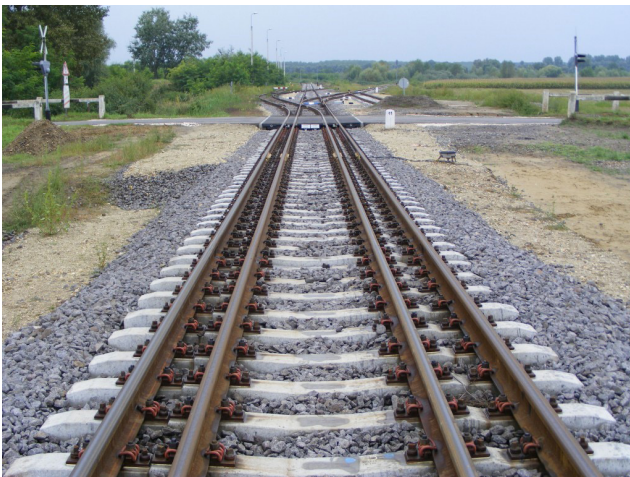
Fig. 3 Construction of crossing and switch interchange on the dual gauge line (Hungary) (NIF Zrt., 2015)
