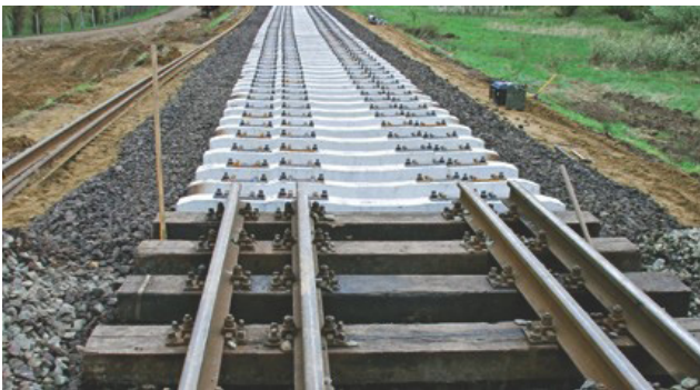
Fig. 2 Repair of the dual gauge line with the replacement of wood sleepers with reinforced concrete ones (Geosynthetic Kft., 2012)
