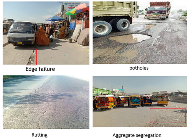
Fig. 13 Road surface issues
